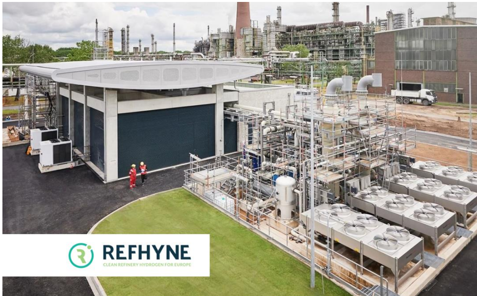
The REFHYNE electrolyser is currently providing renewable hydrogen supply at Shell's Rheinland refinery
